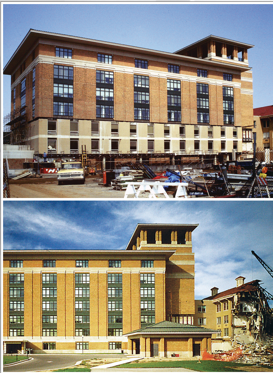
Above: The Murphy Tower is refaced in 1992 during the expansion and remodeling. Below: The original hospital structure is razed in 1993.
